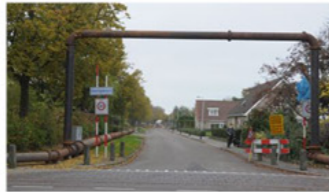
Pipes above ground
