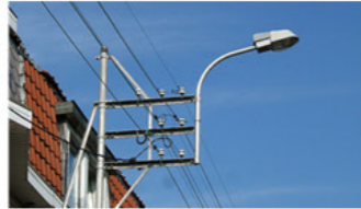
Cables above ground
